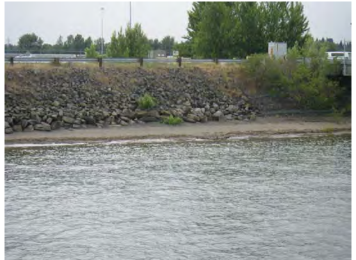
Photo 4: Existing Bank Conditions
