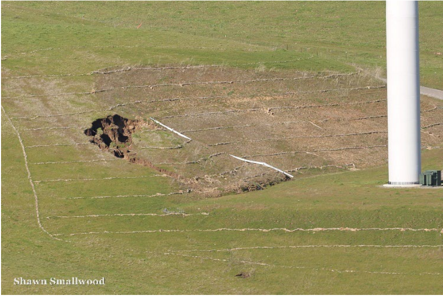
Photos 3 and 4. Soil erosion in wind projects often originates at the corners of turbine pads (top) or on cut slopes (bottom)
