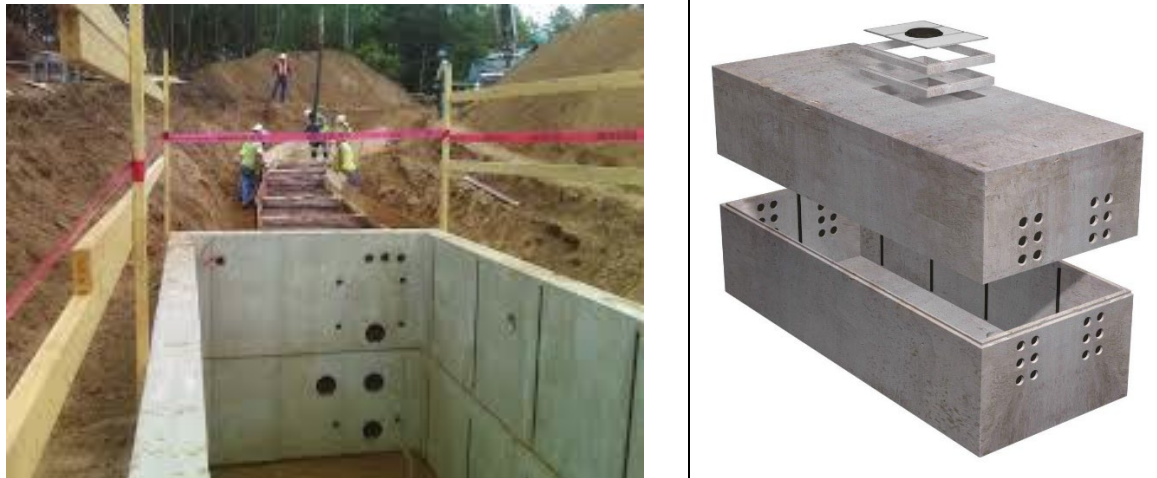
Figure 4: Underground Vault (Xcel Energy 2014, Oldcastle Infrastructure n.d.)
