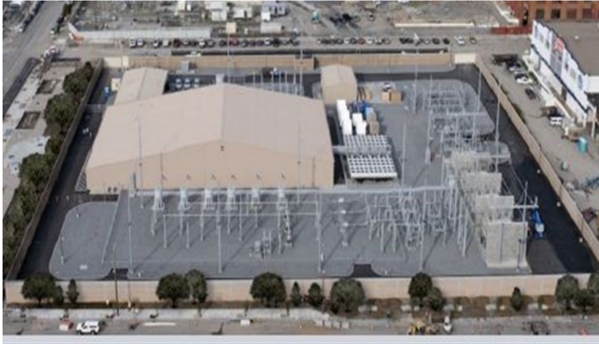
Photo: NextEra's Trans Bay Cable converter station San Francisco, CA
