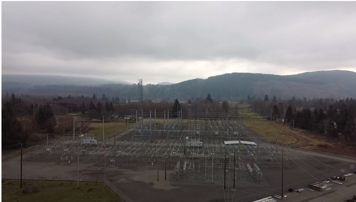
View of Sedro-Woolley Substation from Minkler Road facing South
